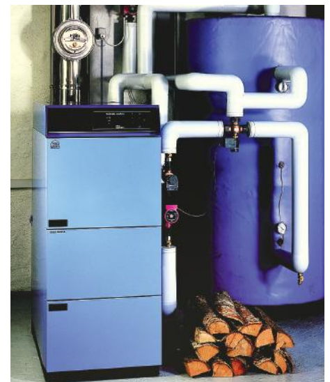
A heat storage system will produce and store hot water throughout the year.
