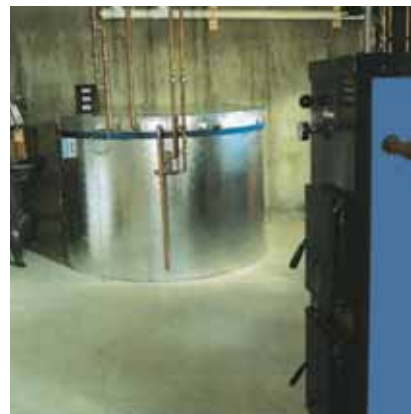
Excel boiler with Storage Tank.
