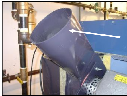
Fig. 3.4 Flue Gas Exhaust Pipe
