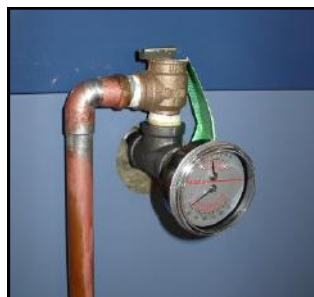
Fig. 3.10 Installed Relief Valve
