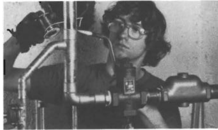
Air purger, valves and copper pipes were plumbed and soldered according to the manufacturer's recommendations.
