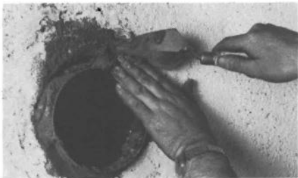
Before flue pipe was passed through wall, thimble was mortared in place. Then flue pipe was inserted and the joint sealed.
