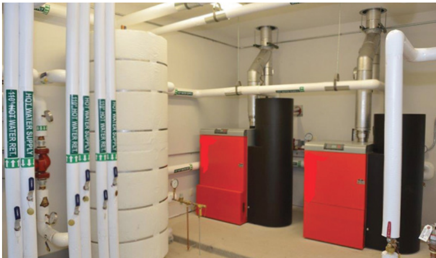
FIGURE 14: Example of two small pellet boilers (red) coupled with a thermal storage tank (large white insulated tank on left).
